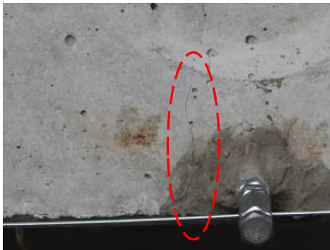
Figure 9 – Occurrence of the first cracks near the average cross section at a total load of 163 kN, such as pre-stressed PNC
