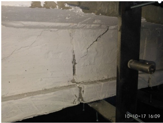
Figure 6 – Inclined crack from the top of the artificial normal crack in the beam
