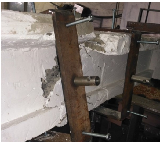
Figure 7 – The destruction of the beam
